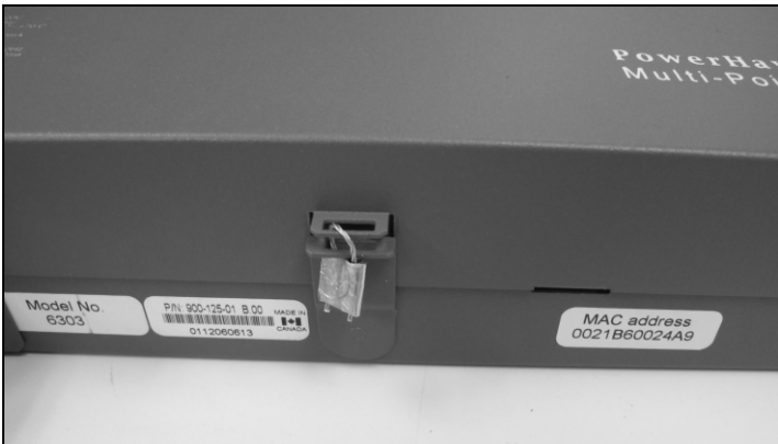
Utility Sealing Location / Emplacement du sceau du service public.
