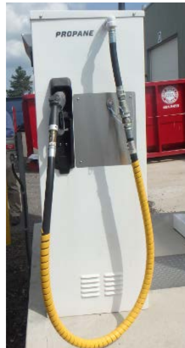
Figure 7: Propane dispenser (Profile view) / Distributrice de propane (vue de profil)
