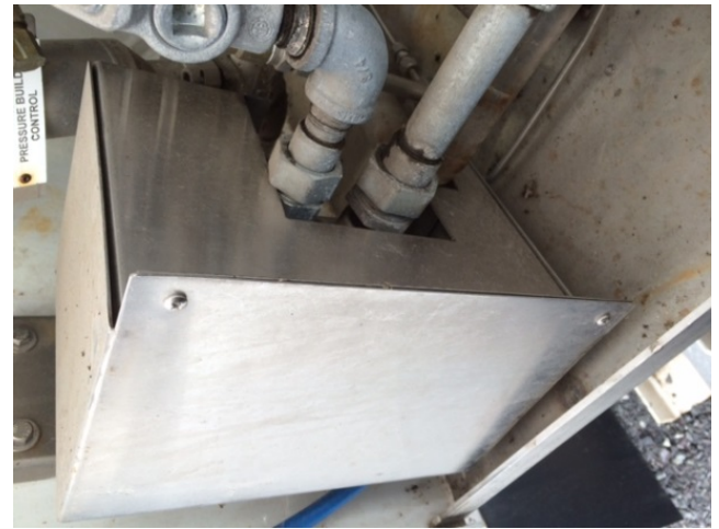
Figure 3 : Cabinet to allow sealing of remote junction box to the MDV 3700 Transmitter / Cabinet permettant le scellage de la boîte de jonction distante du transmetteur MDV 3700
