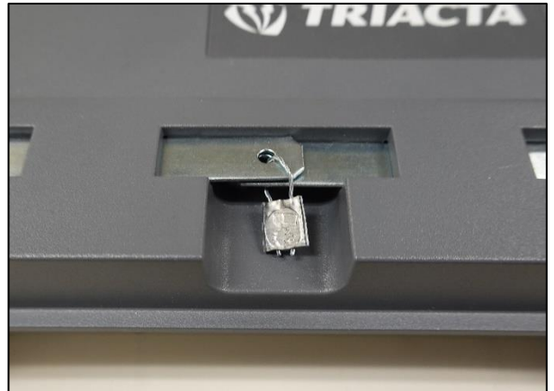
Utility seal / Sceau de service public
