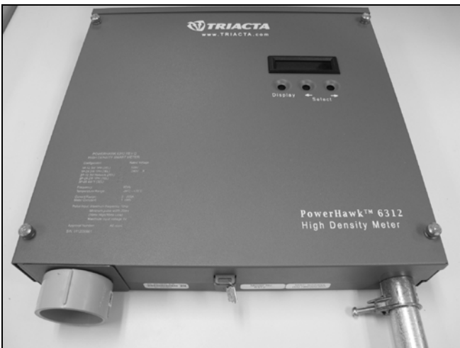
(2) Utility Sealing Location / (2) Emplacement du sceau du service public
